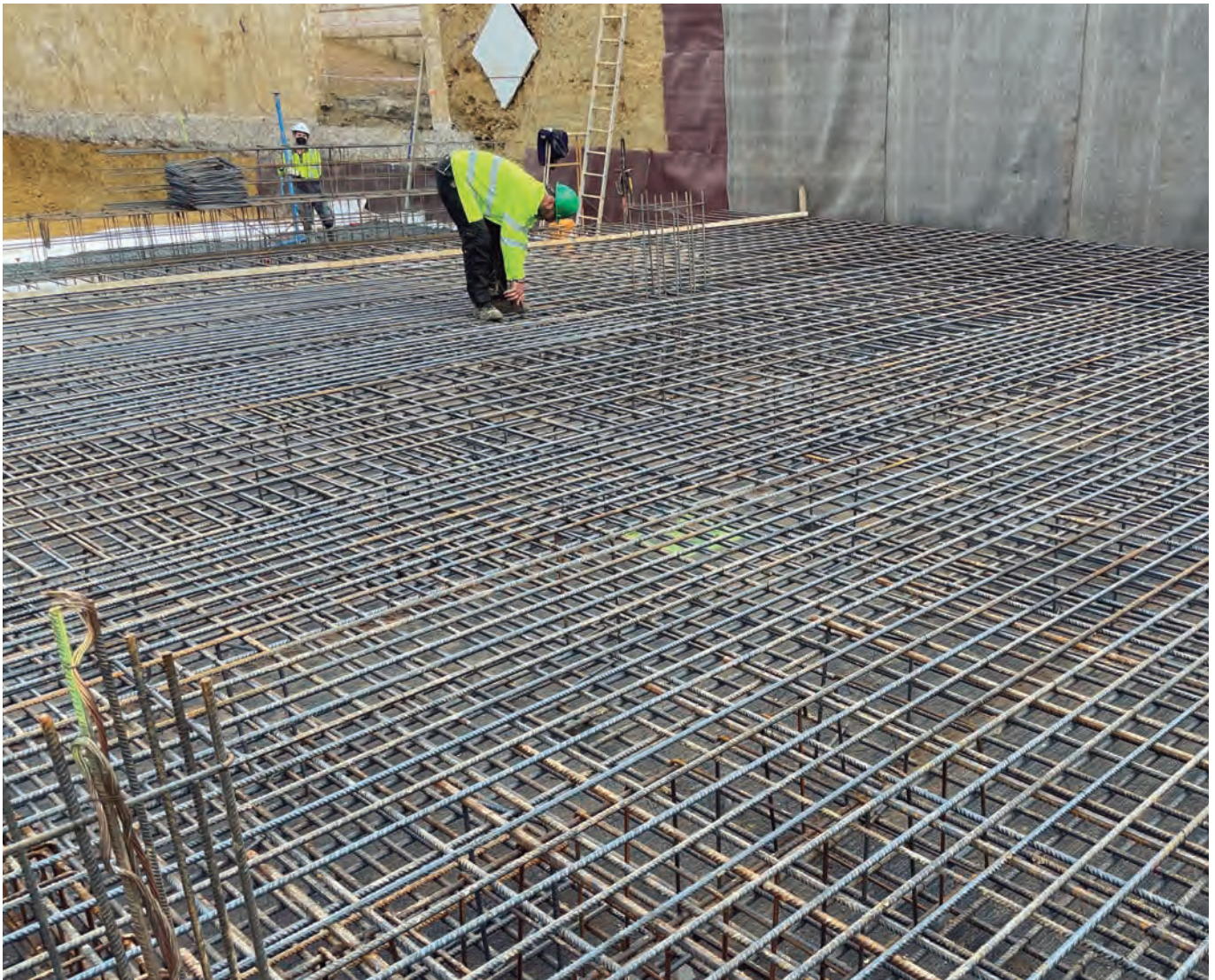
Picture: Construction work at an Arqura Homes residential property development in Huelva (Andalusia).
